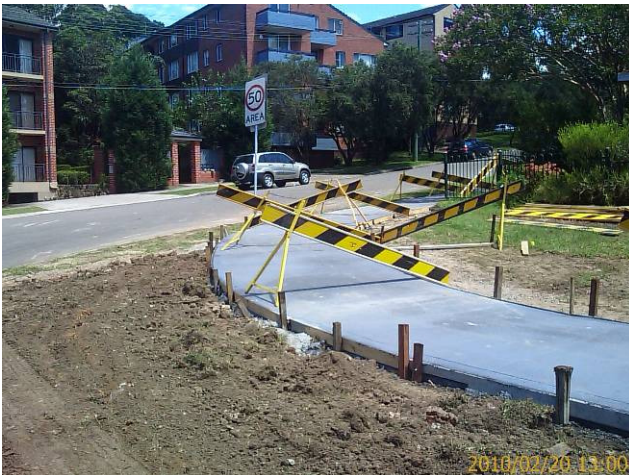
Corner on path is too tight
